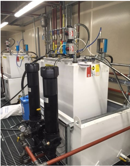
Hydraulic reservoirs with LMD 431 in-line duplex filters
